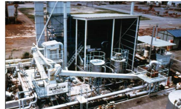
COM (coal-oil-mixture) pilot plant for which Kawasaki developed production facilities and boilers (1980)
