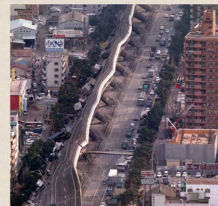
Expressway collapses during the Great Hanshin-Awaji Earthquake
