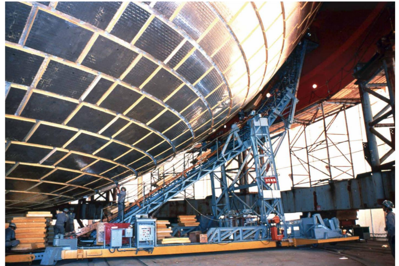
Construction of Kawasaki Panel System, Kawasaki's proprietary insulation system for LNG carrier tanks
