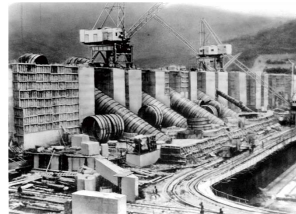
Installation of penstocks (built in 1944) during construction of the Songhua River Power Station (Manchuria)
