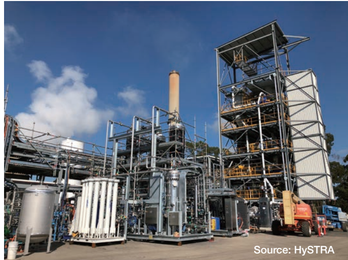
Fig. 6 Brown-coal gasification and hydrogen refining facility (February 2020)
