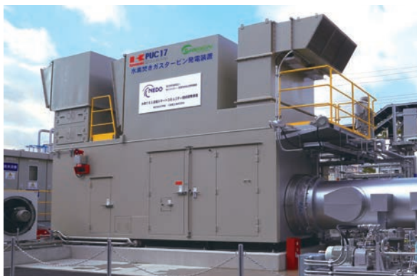
Fig. 10 Cogeneration facility with flexibility in the fuel mixing ratio of hydrogen to natural gas
