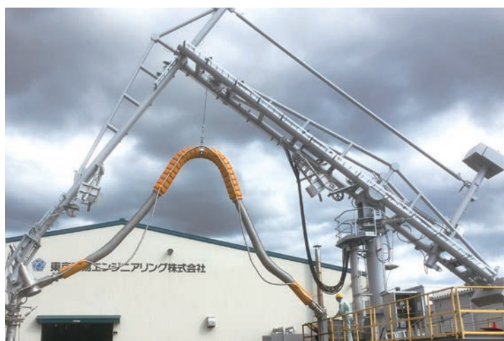
Fig. 6 Loading arm systems for demonstration project
