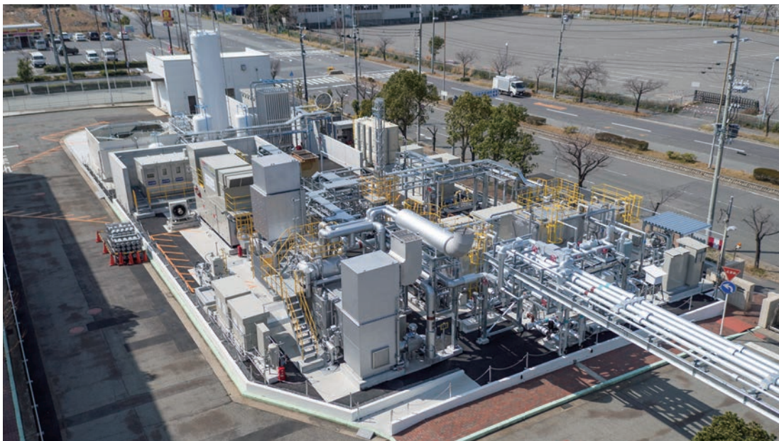
Fig. 5 Demonstration facility for hydrogen fueled gas turbine cogeneration (in Kobe City)
